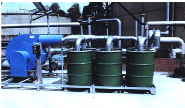
Oil Tank Vent Installation with Six a-SORB™ Canister System
