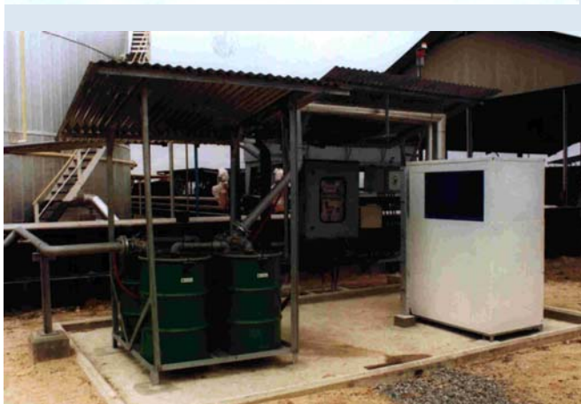
Chemical Plant Installation with Quad a-SORB™ Canister
